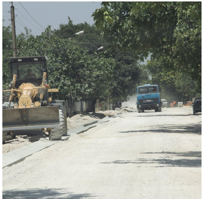
Renewal of the main road in the village (Zone B) (Hanns Kirchmeir)
